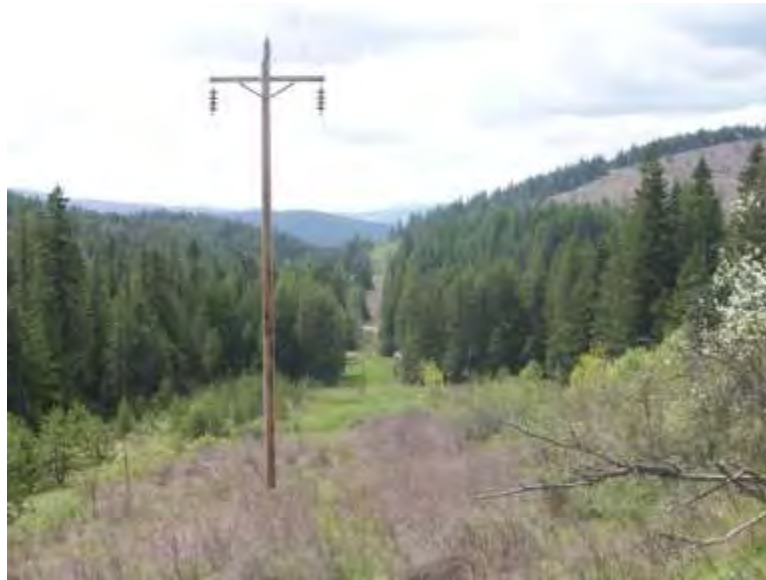
Figure 72. Well-maintained power line corridor between Emida and Sanders.
