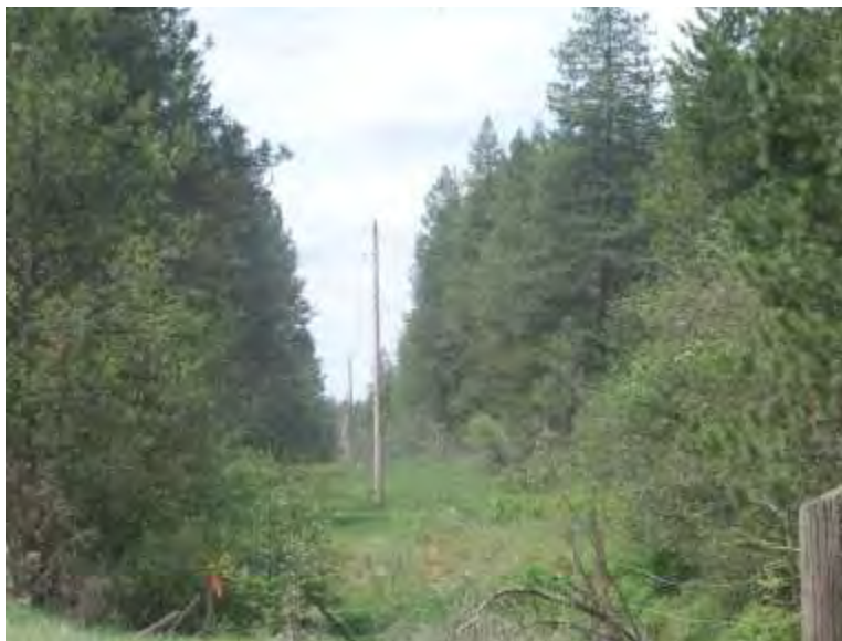
Figure 142. Good power line protection between Sanders and Emida.
