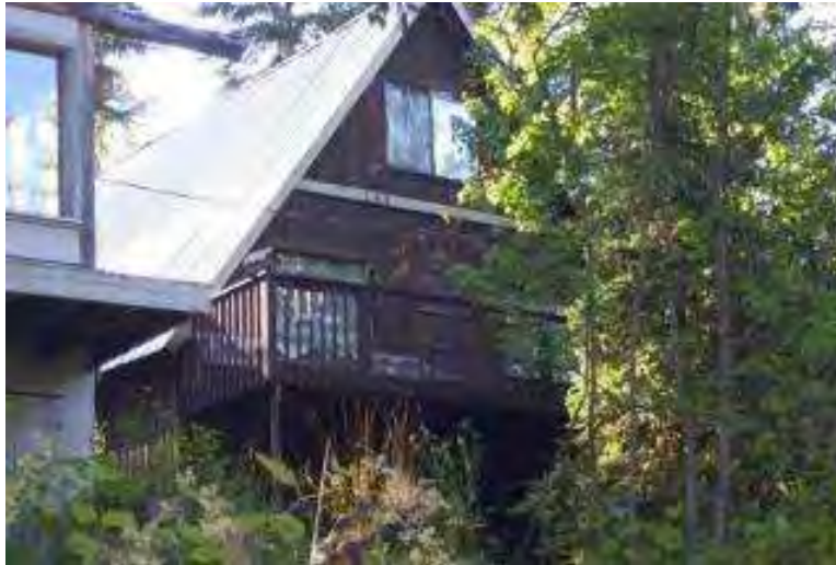
Figure 58. Home built with metal roofing, but wooden siding and deck with vegetation growing against the structure; in need of defensible space.
