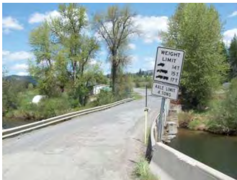
Figure 100. Bridge weight-limit signage accessing Carpenter Creek.
