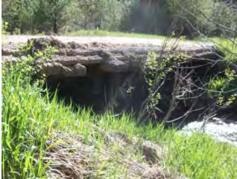
Figure 45. Access bridge to Alder Creek from Benewah Valley Road, needs weight posting and guard-rails.
