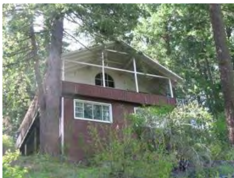
Figure 56. Home with vegetation growing against structure, in need of defensible space.
