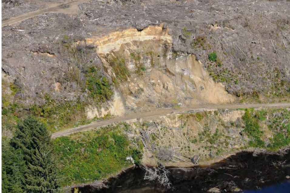
Figure LII. This landslide (Winter 1997/98) on the 7000 Road near Taholah along the Quinault River endangered the Taholah village's water system at Shale Slough (Workman 2009).
