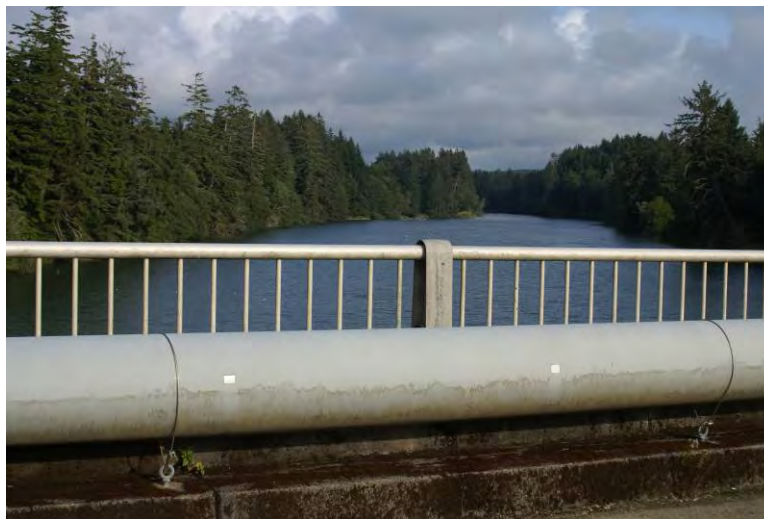
Figure CXVIII. Water Supply Pipe Supported on the Taholah/Quinault River Bridge.
