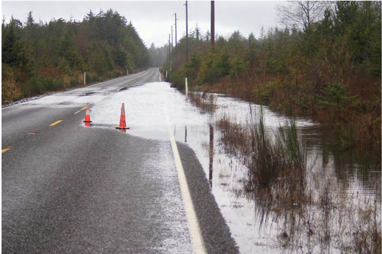
Figure CXXI. One of the infrastructure failures on the QIR in need of mitigation measures. This one is along SR 109 between Moclips and Taholah and is the only access route in and out of the QIR's largest population center: this picture was taken after a moderate rainfall system hit the area.
