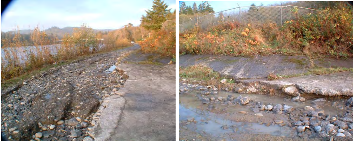
Figure LXXIX. Queets River flood inundation to the access road from the Village of Queets to the Queets Rose Bowl (waste water treatment facility) (Wells 2010).
