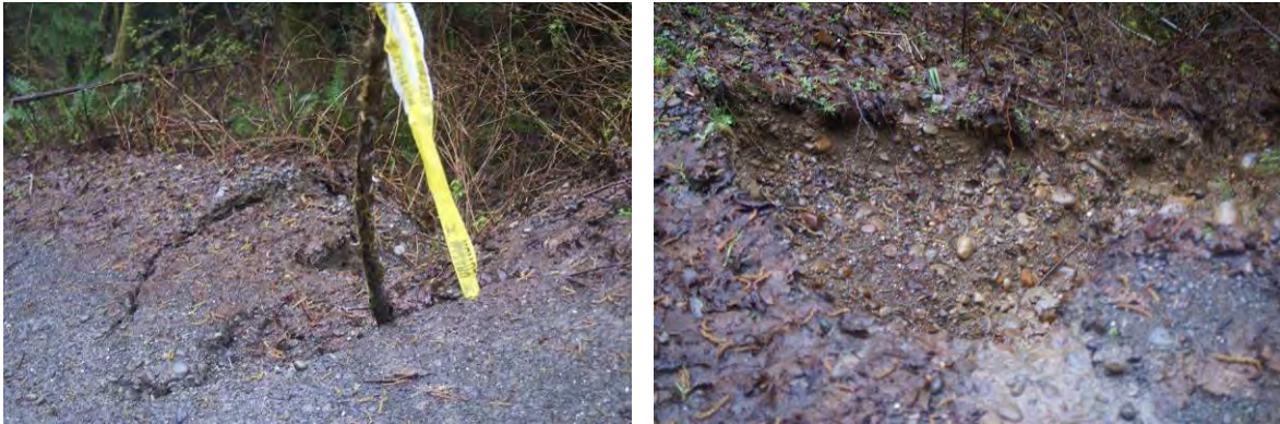
Figure XXIX. Characteristic slumping of a QIR forestry road on the outer edge of the lane where small diameter gravels of the road base have been washed away.
