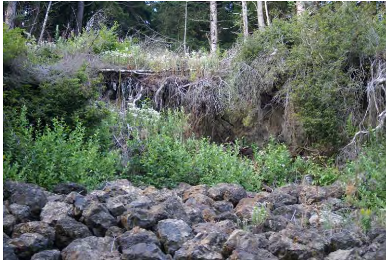
Figure LI. Shallow Undifferentiated Landslide on the uphill side (northeastern side) of SR109 at Swede Hill.
