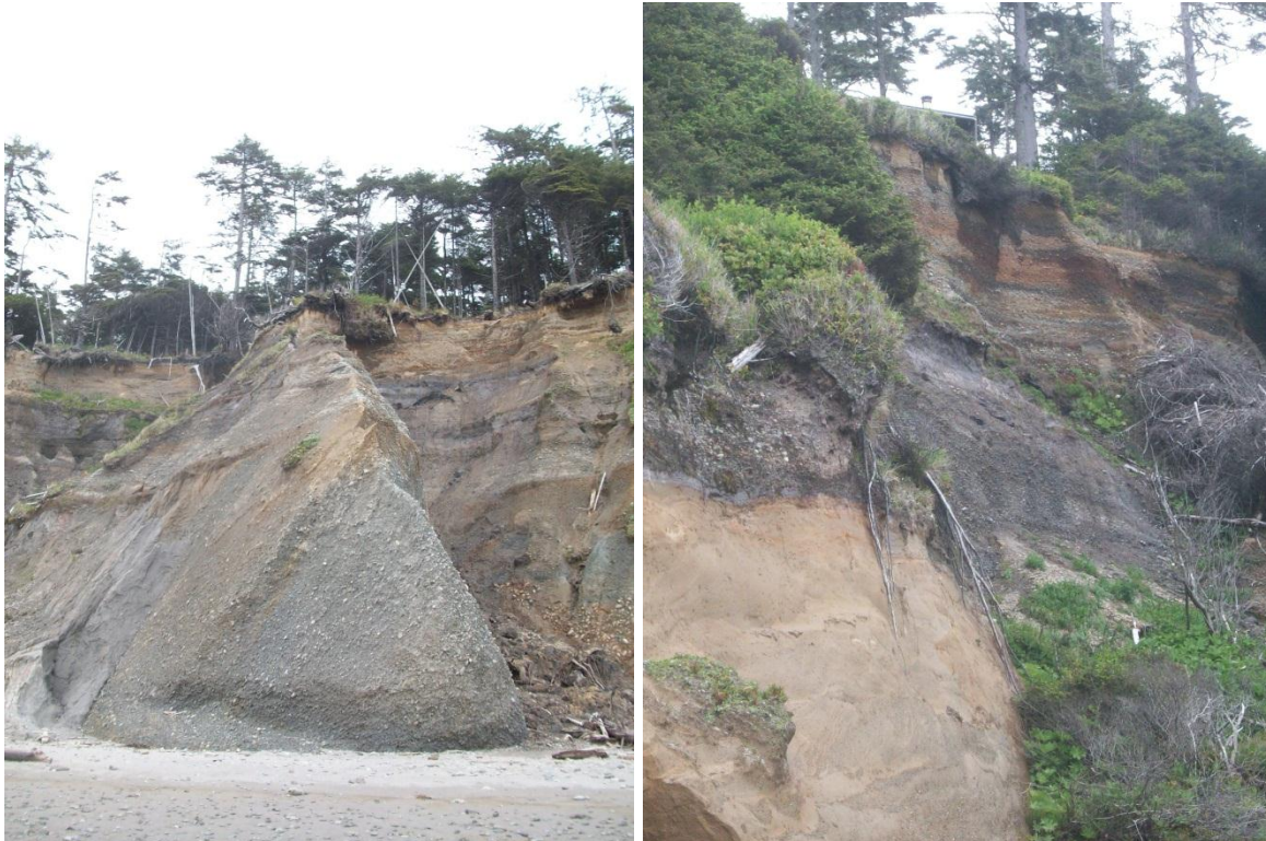
Figure 66. Sand and gravel cliff faces common in the cliffs surrounding Whale Creek.
