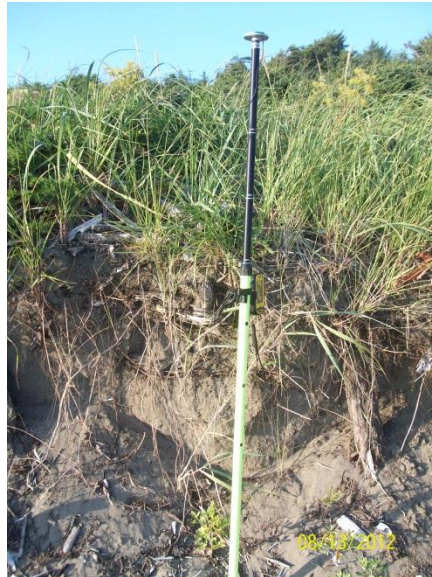
Figure 18. Avulsing CRLC sands north of the Moclips River along the Grenville Bay shorelines; staff is 2 meters tall, sand loss is about 1 meter in depth.
