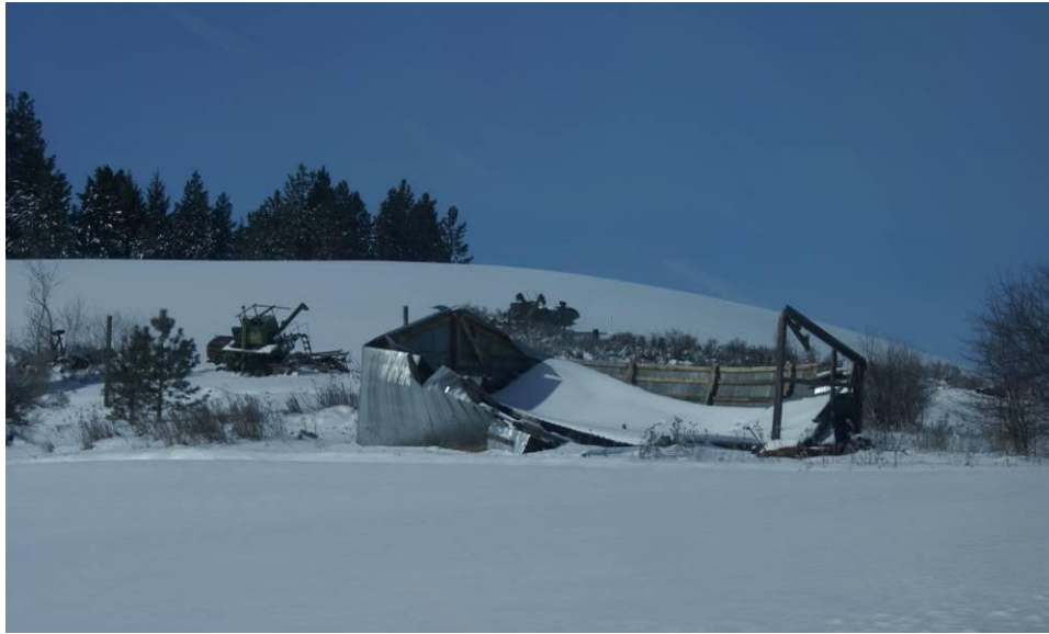
Figure XXXIX. Structural collapse under snow load along US 95, south of DeSmet and north of Sanders in February 2009.
