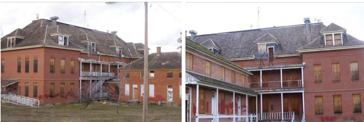
Figure LXVII. Sister's House in DeSmet – URM and condemned.
