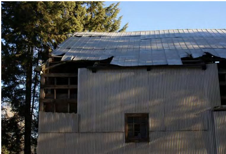
Figure LXXXIX. Example of windstorm damages to a structure near Rocky Point, on State Highway 5, west of St. Maries.
